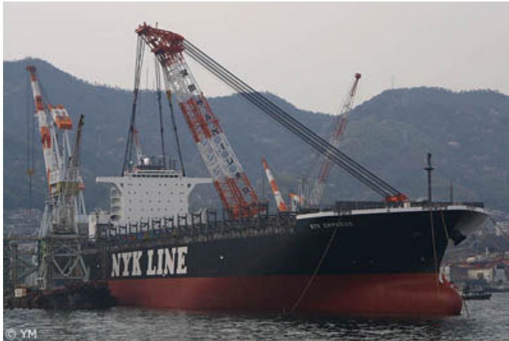
At IHI's Kure dockyard in Japan, the superstructure is lifted onboard the new 9,200 TEU vessel NYK Orpheus. photographer: Y.M. (anonymus)
